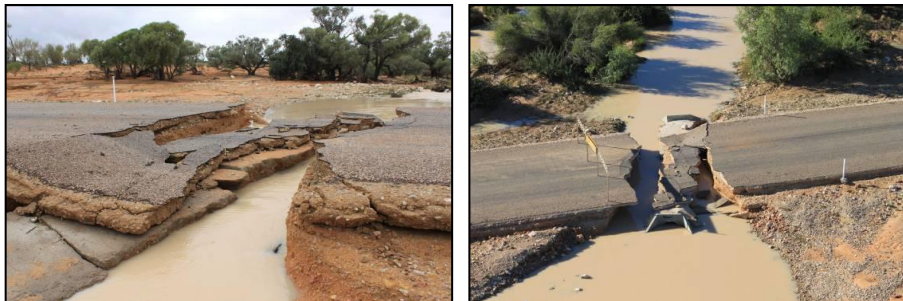
Figure 2: Flood damaged roads in Central West Region, Queensland, Australia in early 2011[3]
